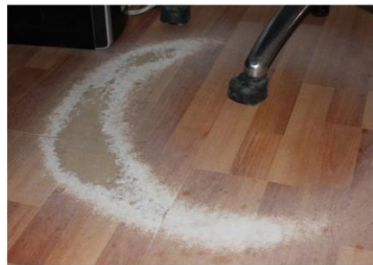
Wrong laminate category
