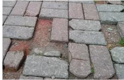
Wrong paving blocks
