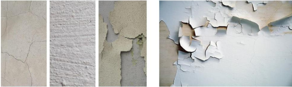
Wrong putty type
