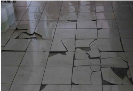
Wrong outdoor tile
